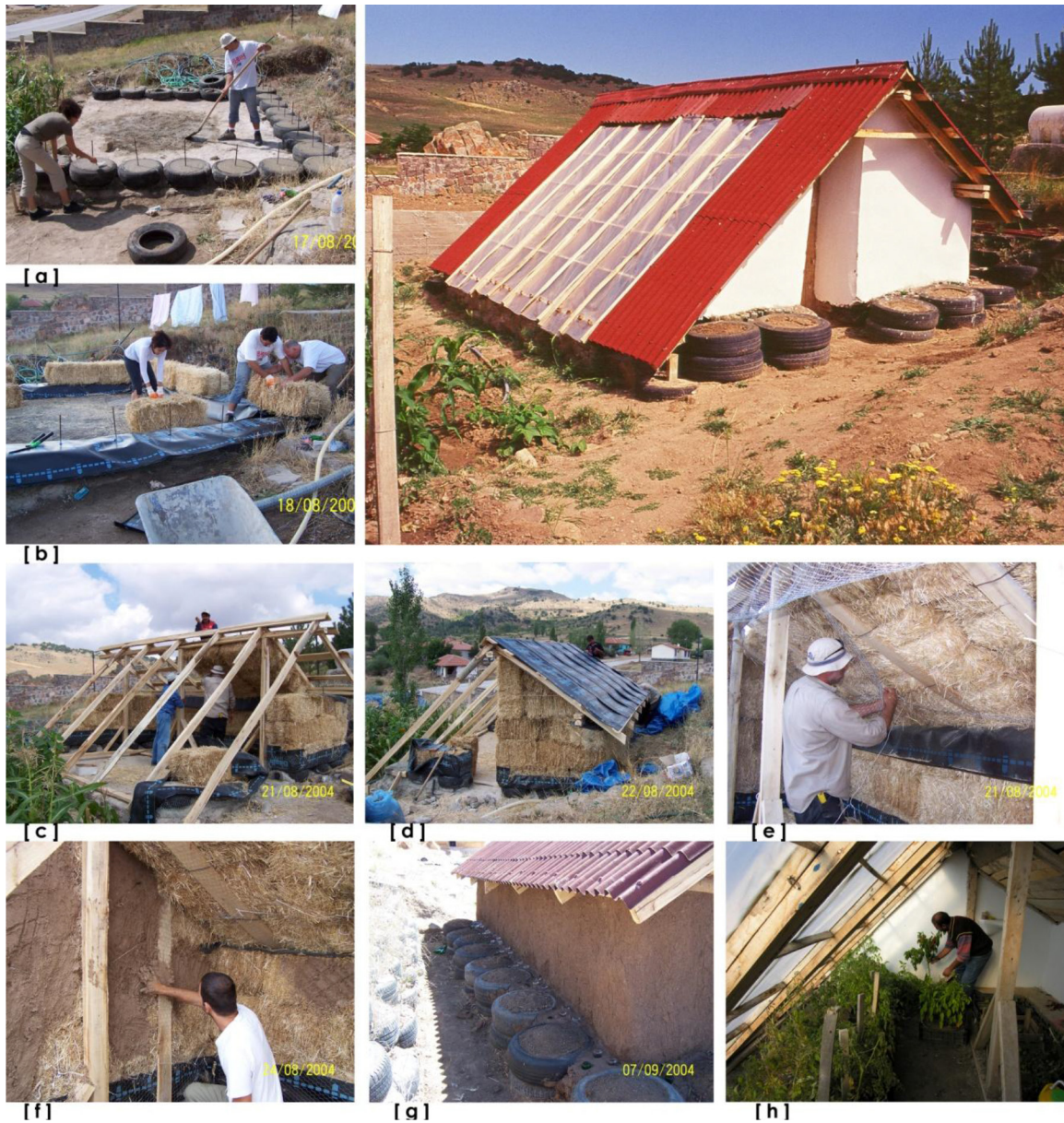
FIGURE 1. The Strawbale Greenhouse: [a] laying the foundations; [b] anchoring the first row of strawbales for the walls; [c] erecting the wooden structure; [d] roof insulation; [e] sewing on the chicken-wire before mud-rendering; [f] plastering the bales with mud and straw mixture; [g] plinth protection made of old tires, bottles and mud; [h] interior of the greenhouse.
