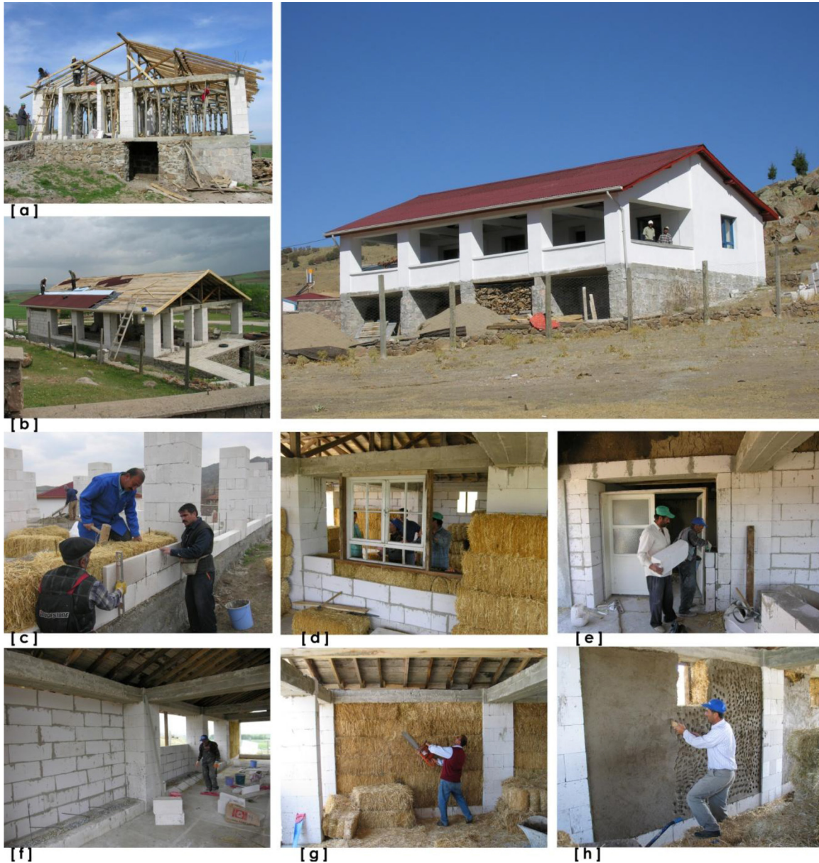
FIGURE 5. The Strawbale Conservation Workshop: [a] timber roof structure, concrete lintels and AAC piers on stone foundations; [b] laying layers of insulation on the roof; [c] wall composed of strawbales and AAC blocks; [d] installing a re-used door; [e] installing a re-used door; [f] interior view of external layer of AAC blocks; [g] trimming the straw bales; [h] plastering interior wall surface with mud and straw mixture.
