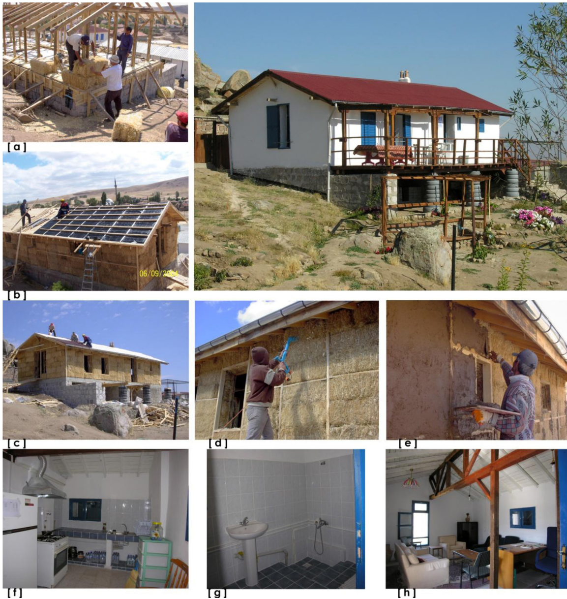
FIGURE 3. The Strawbale House: [a] Timber structure on stone foundations; [b] erecting the roof structure; [c] finishing the roof; [d] trimming the straw; [e] applying mud-plaster on the walls. [f] The kitchen; [g] bathroom; [h] and interior of the strawbale house.
